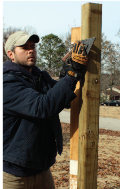
Use a story pole to mark your stringer locations along the posts.
