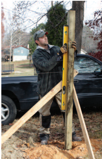
A traditional method to plumb and brace posts is to use a 4-foot level and a couple of pivoting wood legs.
